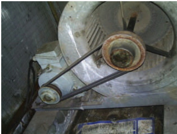
The AHU Showing the Motor and the Belt Drive.
