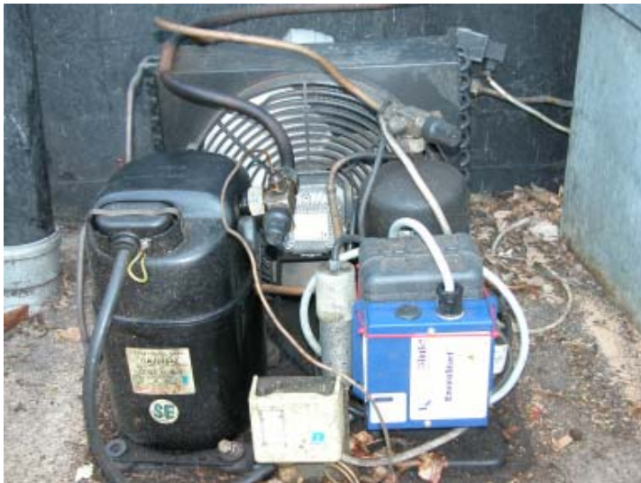
External Refrigeration Chiller
